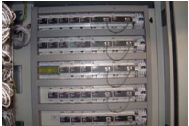
At the Biopolis, Dupline controls and monitors more than 1,500 ACMV equipment such as exhaust fans, AHUs, FCUs, all over normal two-wire cables.
